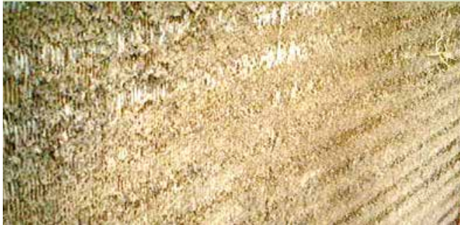
Dirty Coil Before HVAC Tune-Up
