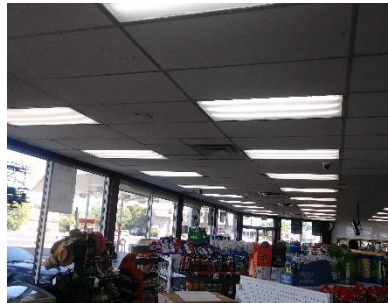
Figure 1.2 (Sample picture of ceiling fixtures)
