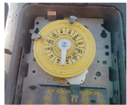
Figure 1.12 (Sample picture of a control device)
