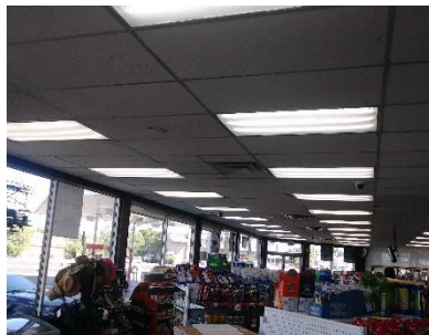
Figure 1.2 (Sample picture of ceiling fixtures)
