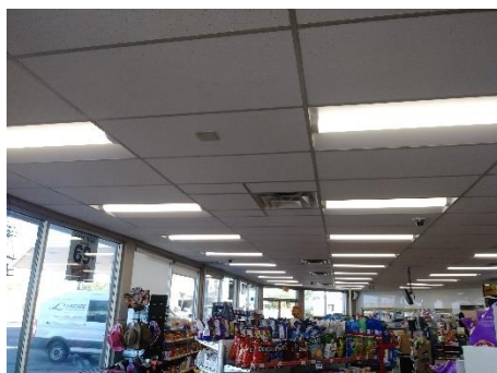
Figure 1.14 (Sample picture of ceiling fixtures)
