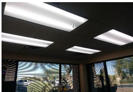
Figure 1.1 (Sample picture of ceiling fixtures)
