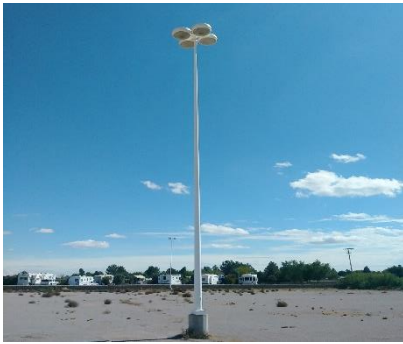
Figure 1.7 (Sample picture of Pole lighting)
