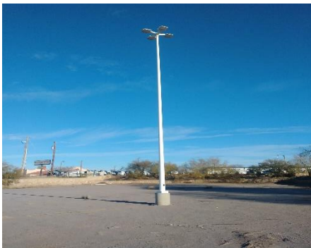
Figure 1.19 (Sample picture of Pole lighting)
